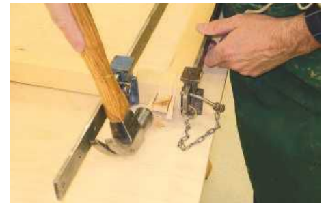
▲ Pic.19 Vertical glazing bars should always run the full height of the sash and be through tenoned and wedged at meeting rails
